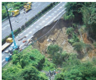
Immediately after the earthquake (August 2009)
